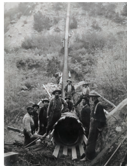
Water Pipe Nettle Creek: "Workers construct the diversion tunnel that will bring water from Nettle Creek to Carbondale's municipal water system." DeBeque Collection photo
